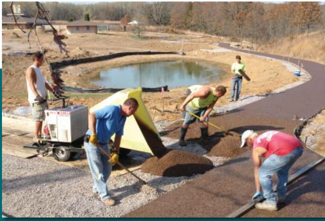
Workers from Vinton Construction Company, Manitowoc, WI, level open-grade base course and install the top layer for a FilterPave path at the International Crane Foundation in Baraboo, WI
