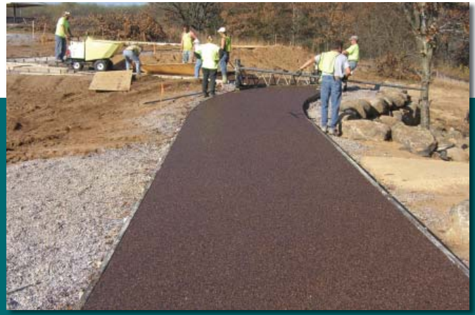
A completed section of path shows the color and smoothness of the finish. Water percolates through the pavement into the ground, where it is returned to the water table naturally.
